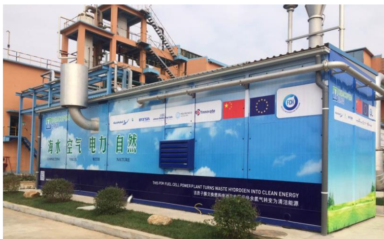
One of the DEMCOPEM-2MW container at Ynnovate
