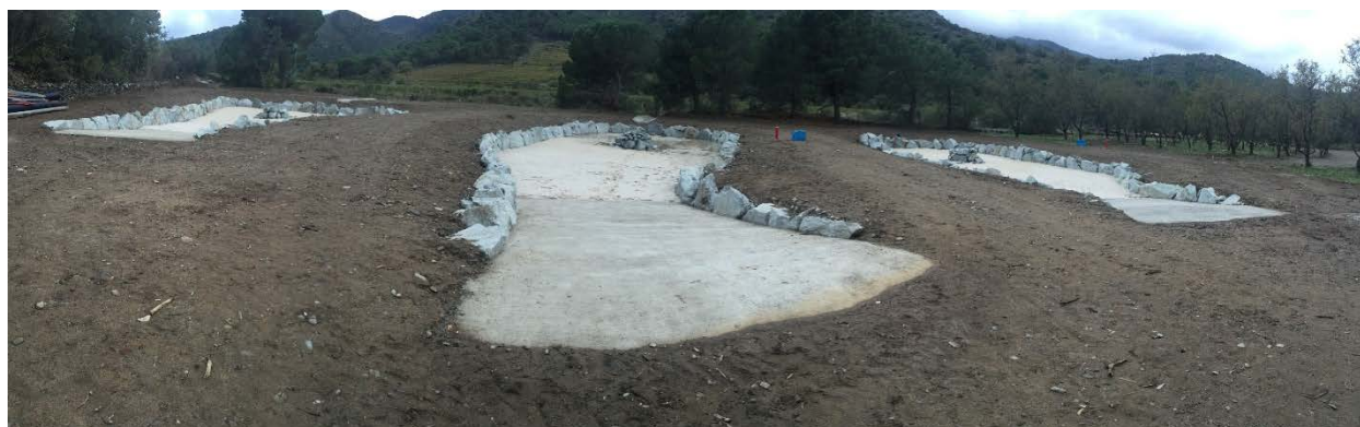
Figure 5 Infiltration basins at El Port de la Selva site
