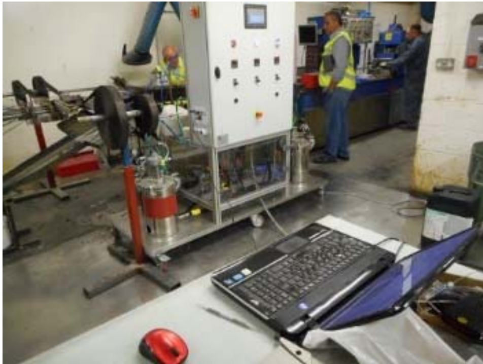
Figure 19. Resin injection system and process monitoring system operating during the installation trial.
