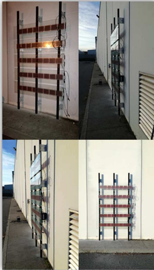
Figure 19 BIPV panels installed on the wall at Onyx in Ávila (Spain).
