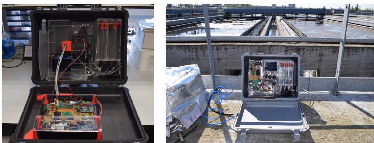
Figure 7 Fully-functioning autonomous nutrient analyser developed by DCU (left) and in deployment (right) at a waste water treatment plant in Milan (organized by UMIL and DCU)
