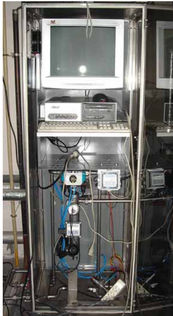
Figure 9 – Details of the EDY system: rack with control PC and probes: prototype installed in Portugal
