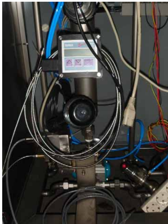
Figure 3 – Details of the EDY system: temperature, pH and conductivity probes /2
