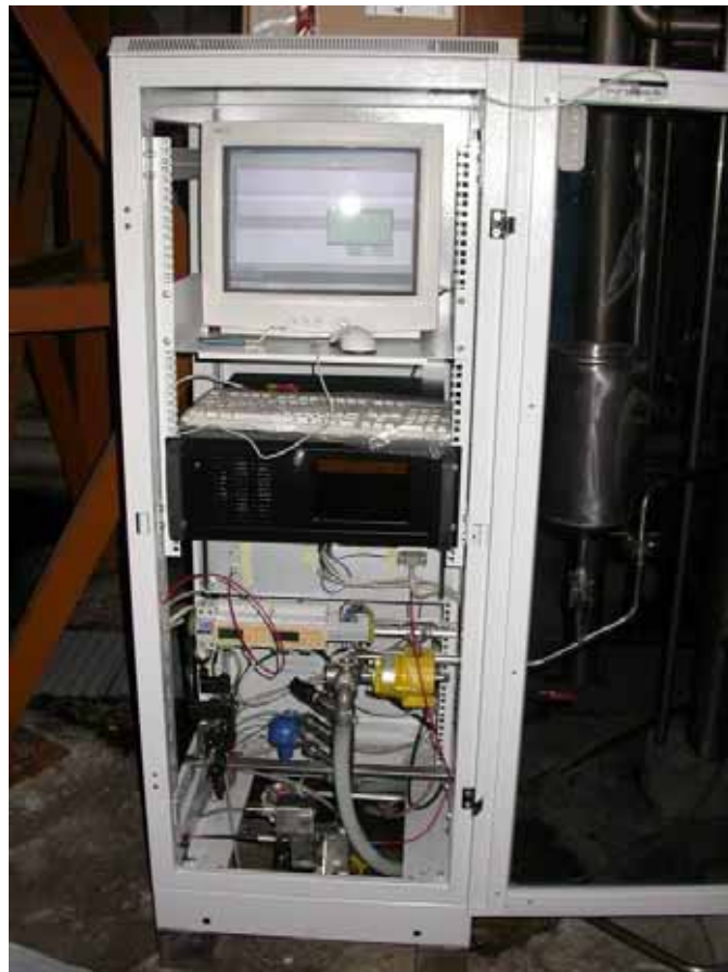
Figure 8 – Details of the EDY system: rack with control PC and probes: prototype installed in Italy
