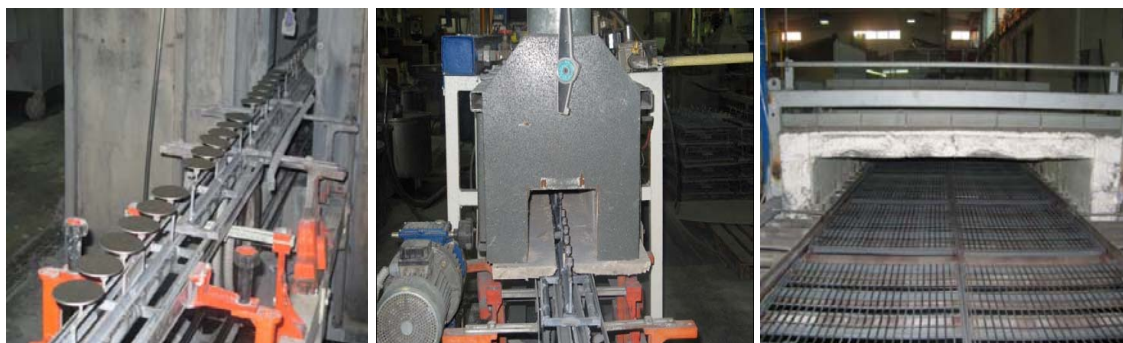
Figure 5. Current burner cap production at Pramur using (from left to right) wet spray enamelling, electric radiation drying and gas-oven enamelling at 850°C.
