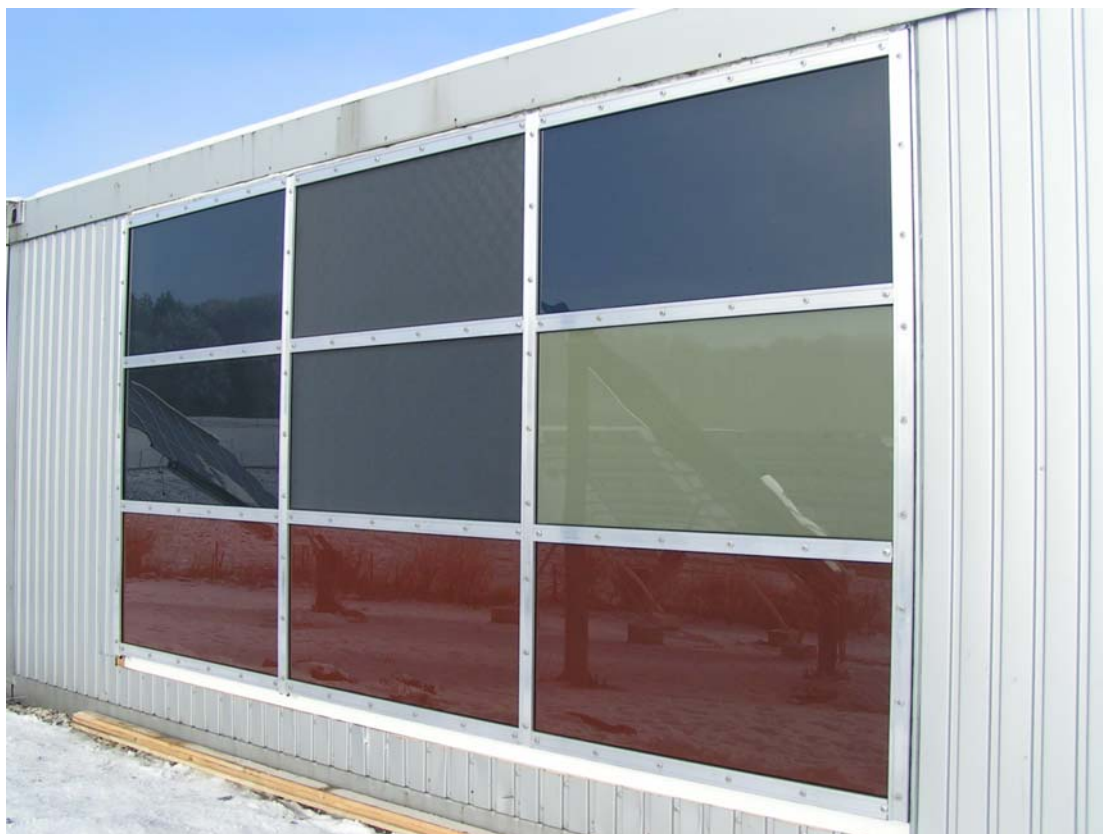
CIS modules, partially coloured, in double glazing units in the transom mullion façade at the ZSW test site Widderstall, Germany. Photo: ZSW
