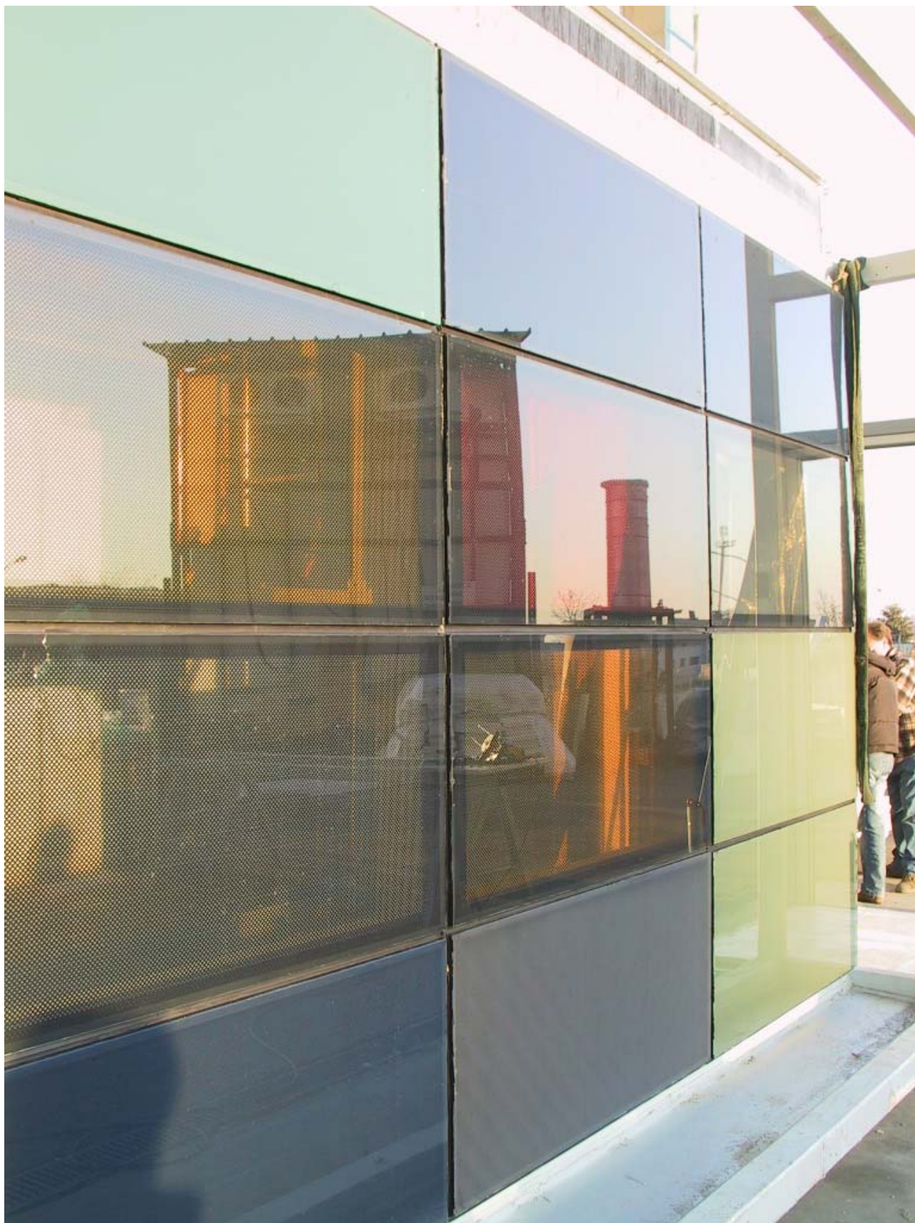
General view of the tested CIS modules modules in double glazing units on a structural silicone frame. Photo: Scheldebouw
