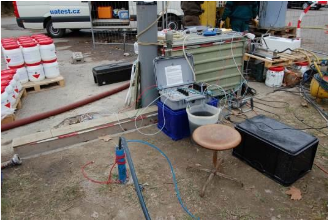
Figure 71: Injection of FerMEG12 (nZVI) into the Solvay site (Source: VEGAS, University of Stuttgart, Germany)
