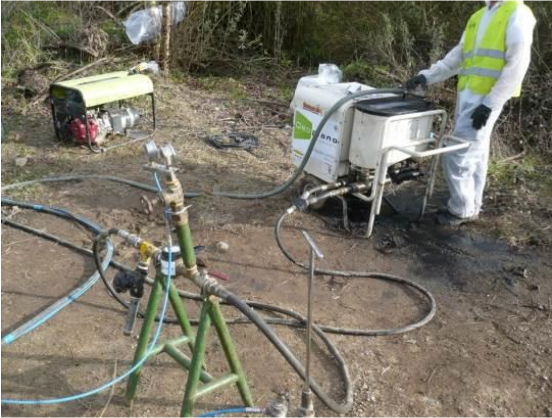
Figure 48: Nitrastur site (Spain): detail of the injection pump, water and pressure gauges used for the injection of nZVI [24.02.2016] (Source: Geoplano Consultores, S.A., Portugal)
