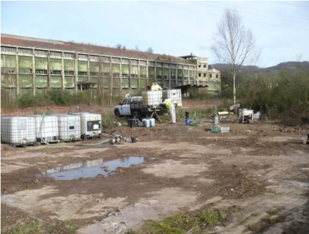
Figure 46: Nitrastur site (Spain): preparatory works for injection of nZVI at the [23.02.2016] (Source: Geoplano Consultores, S.A., Portugal)
