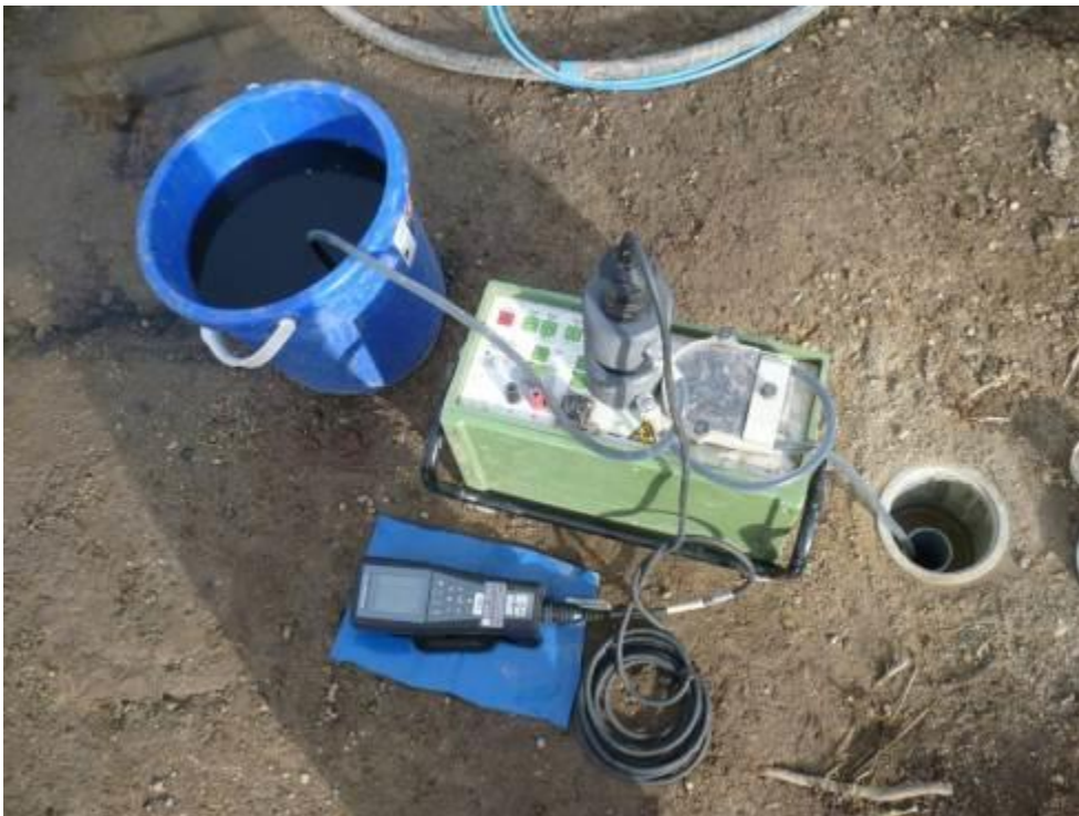
Figure 47: Nitrastur site (Spain): real time monitoring during the nZVI injection [23.02.2016] (Source: Geoplano Consultores, S.A., Portugal)
