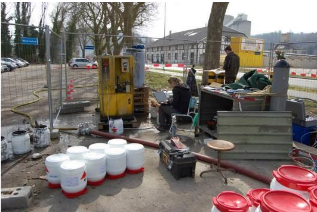
Figure 70: Injection of FerMEG12 (nZVI) into the Solvay site (Source: VEGAS, University of Stuttgart, Germany)
