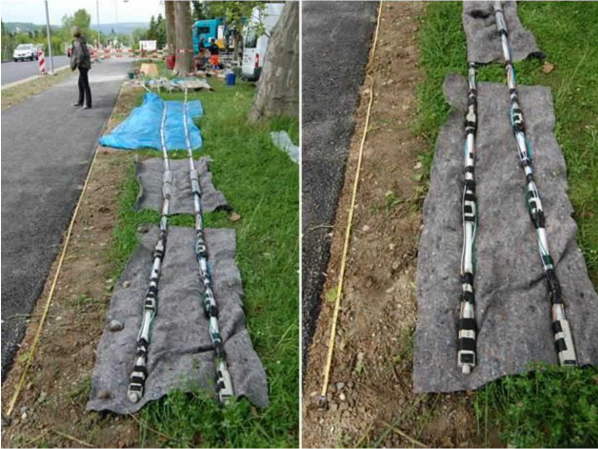
Figure 59: Monitoring arrays for in situ susceptibility measurement ready for installation on pilot site. Configuration and (Source: VEGAS, University of Stuttgart, Germany)
