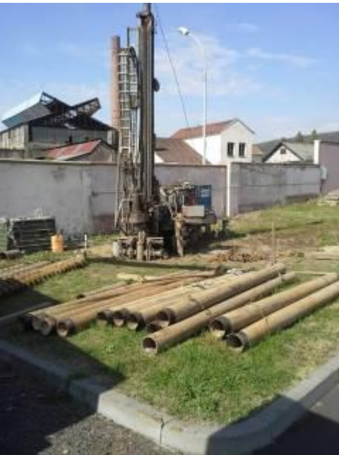
Figure 28: Drilling of boreholes for installation of monitoring system (Source: AQUATEST a.s., Czech Rep.)
