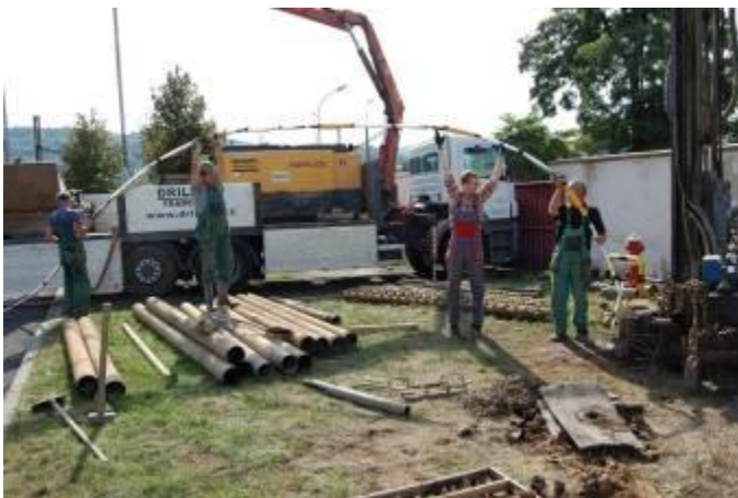
Figure 31: Monitoring system installation (Source: AQUATEST a.s., Czech Republic)
