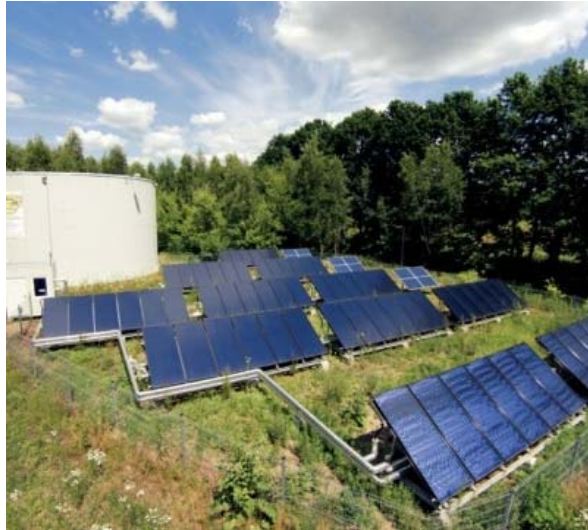
Photo 1. View of the Polish Pilot Plant (STES and solar collectors field)
