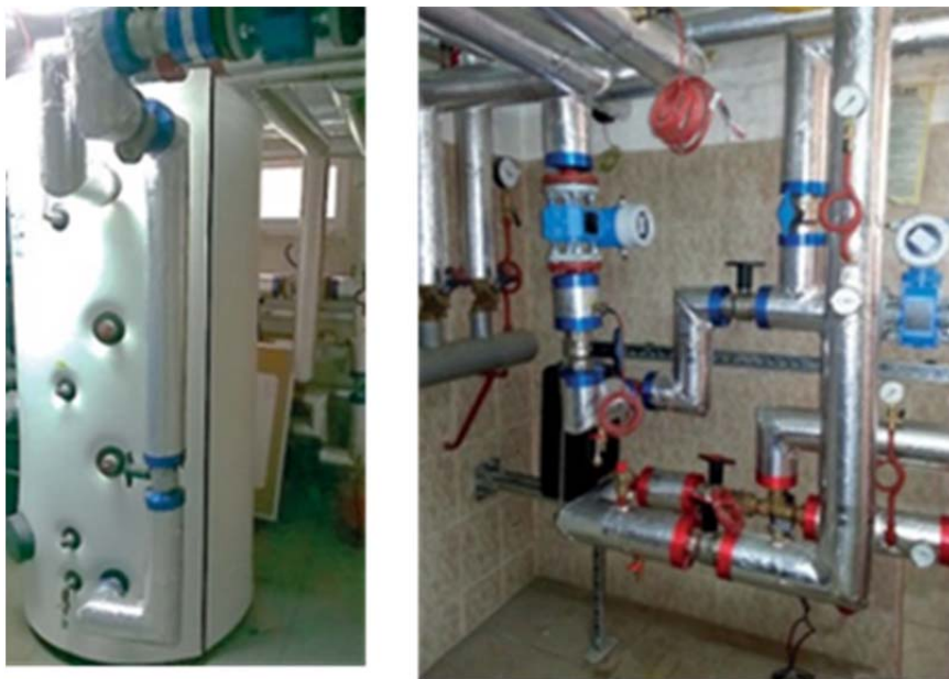
Photo 2. Boiler and its equipment installed room after modernization
