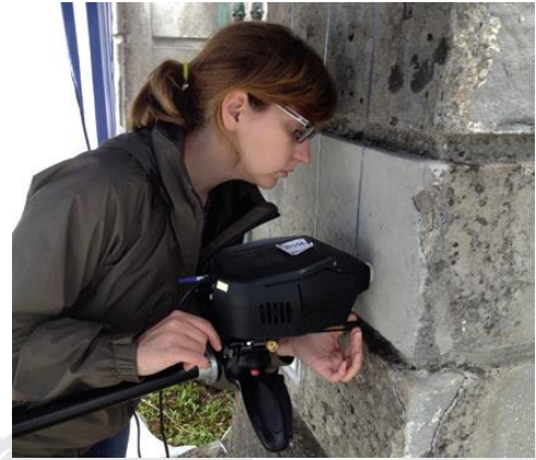
Fig. 16. XRF measurements (non-invasive) to assess the retention of the photocatalytic coating over time, Dornava Manor
