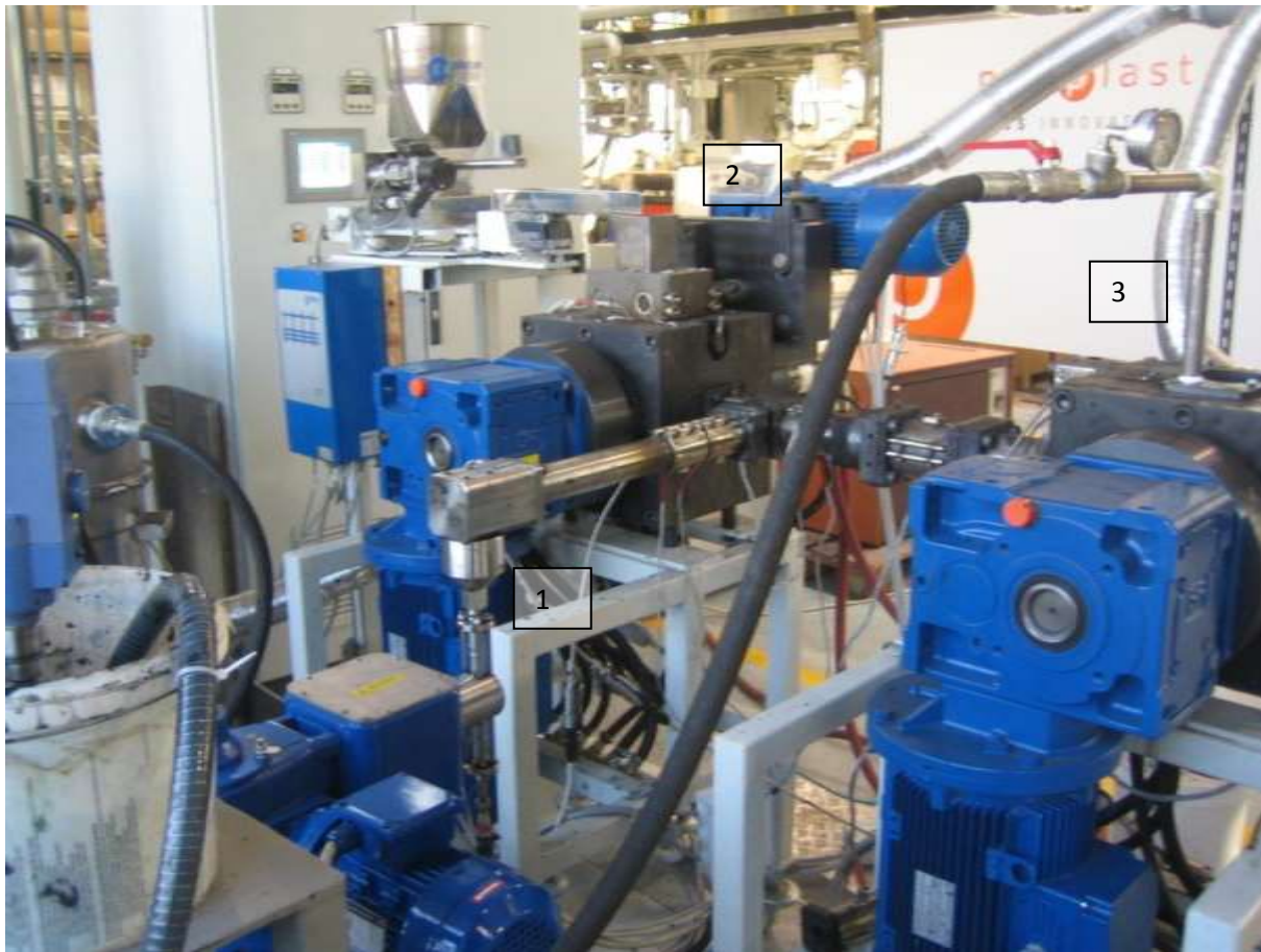
Figure 4.3.2: 1. Nexxus Melting NXBG200W80 ME, 2. Pumping group for the slurry, 3. Nexxus Degassing NXBG200W80 DE
