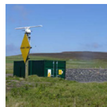
Marine X-band radar system installed at EMEC electricity substation, UK.
