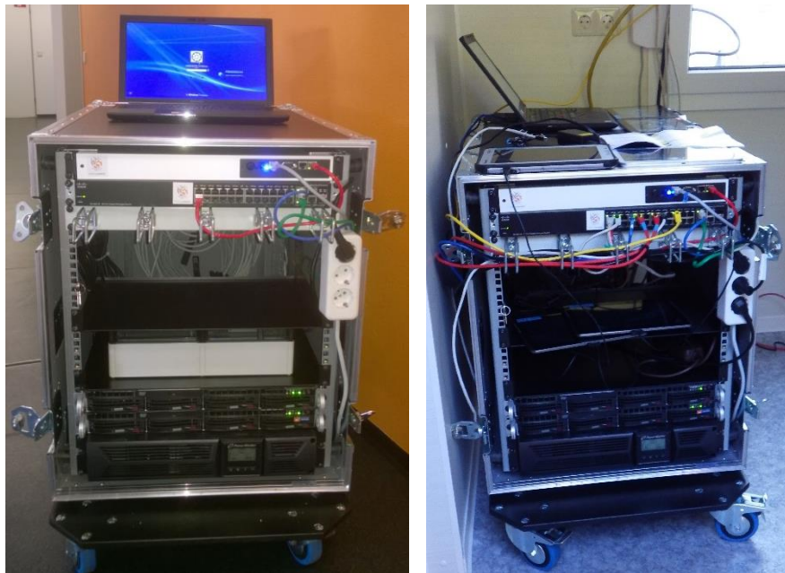
Figure 1: IDIRA MICS server rack
