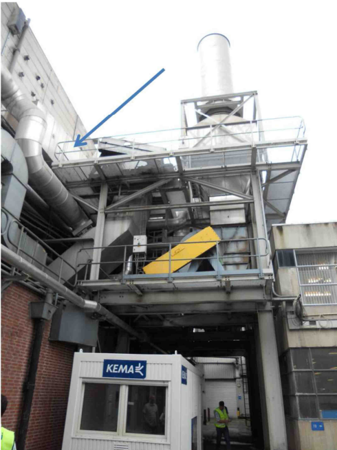
Figure 8 Test location at the dryer exhaust at Sappi Nijmegen
