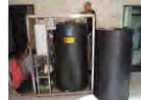
Installation of the MBR pilot plant by IIADEEC Company (Spain)
