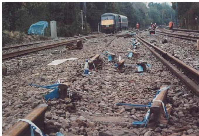
Figure 1 – The Hatfield Rail Track Site following the accident 2
