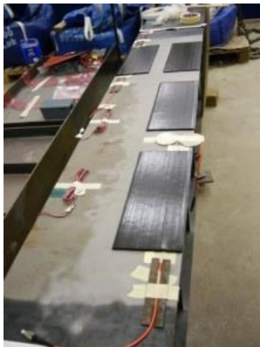
Patch lamination at the bottom flange of a civil engineering application girder
