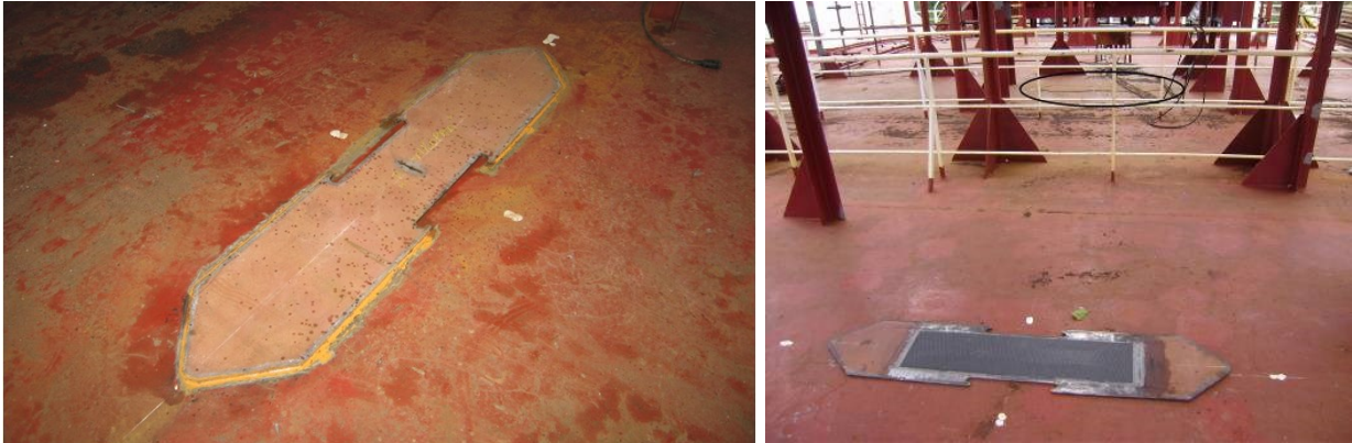
Patch installed on deck of M/V FRANKOPAN – unpatched plate (left), patched plate (right)
