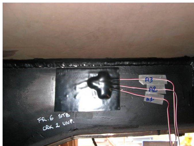
Sensors' wiring at the defects area for monitoring structural response
