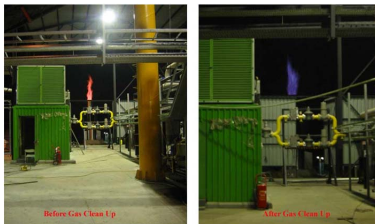
Fig. 21: Flame colour before (left) and after (right) gas clean-up (Source: ITI).
