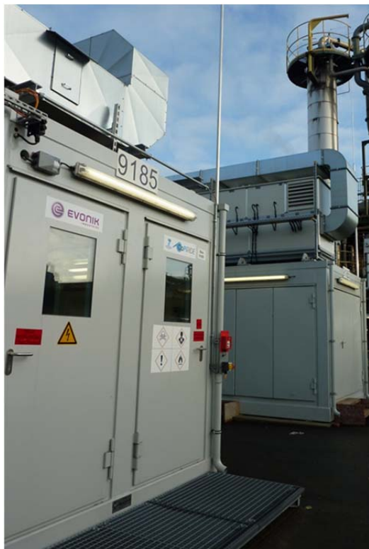
Fig. 7: EvoTrainer plant at Marl side. (Source Evonik)
