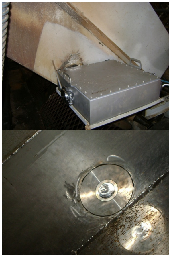
Figure: Integration of the ProFOSS system with the bagasse chute in the sugar mill.
