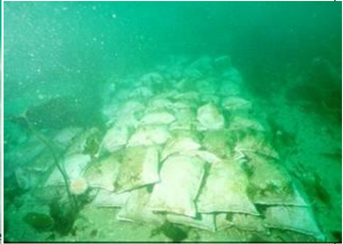
Fig. 7b. Sand bags are an efficient method for securing the sediment layer above the wreck site and establishing unfavourable conditions for biological attack.
