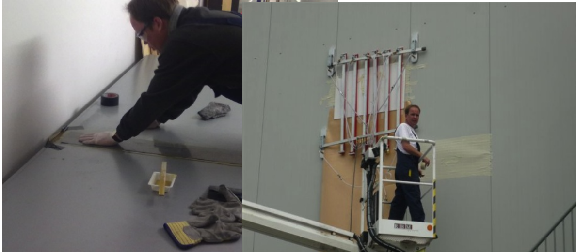
Fig. 4.6: Repairing of artificial defects in the laboratory and real defects on building site by E.Rustemeijer.
