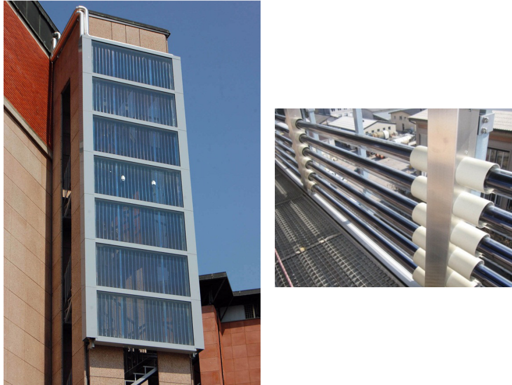
Figure 10 pilot installation in the Slovenian pilot building in Ljubljana. Air heating vacuum tube collectors (right) and transparent solar thermal collectors (left) are used for solar heating and cooling.
