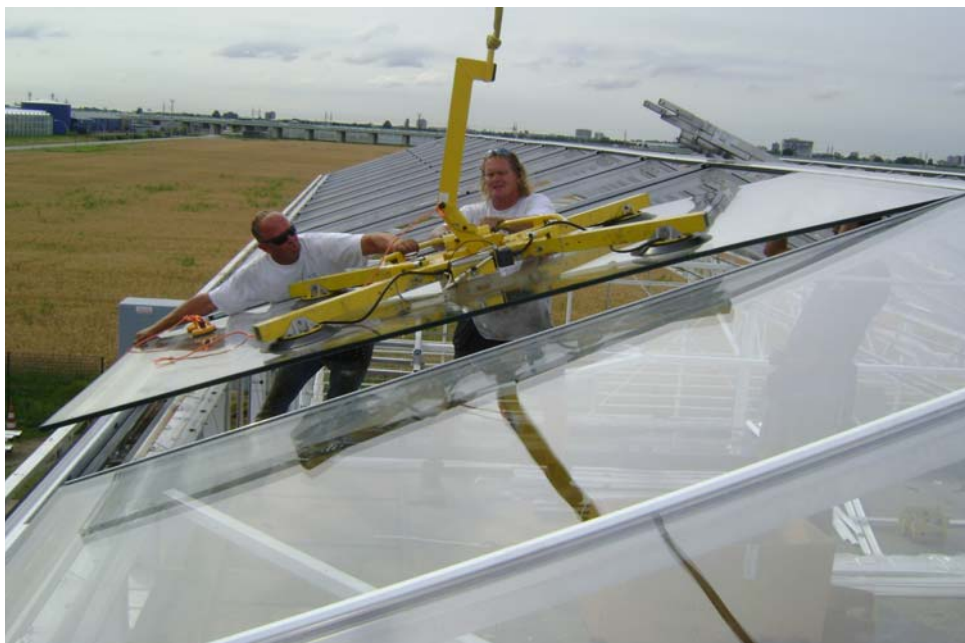
Figure 3. The placing of the innovative double-glass roof on the Venlow greenhouse prototype (co-financed by the Dutch Ministry of Economy and Agriculture and the Dutch Horticultural board). Together with innovative dehumidification, an energy saving of 50% was attained, without loss of production
