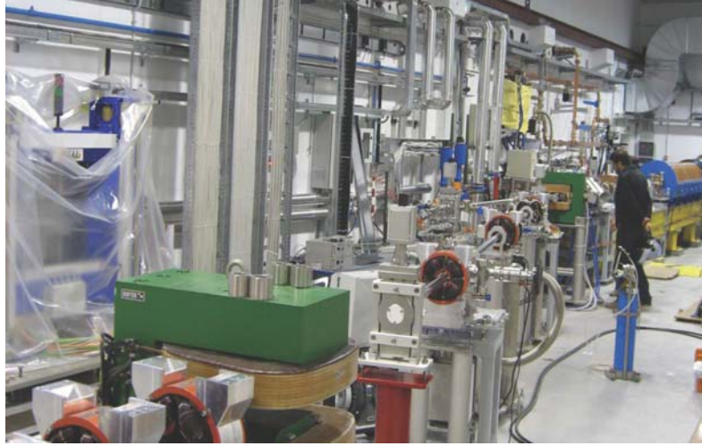
Figure 5: The SPARC facility including the linac with solenoids for velocity bunching (far right), the seed laser injection chicane (middle) and the undulator during installation (left).
