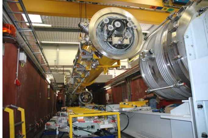
Figure 9: Installation of a 12 m long cryomodule in the CryoModule Test Bench (CMTB) at DESY.
