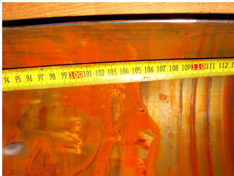
Picture 4.1: Close view of corrosion on the liner.
