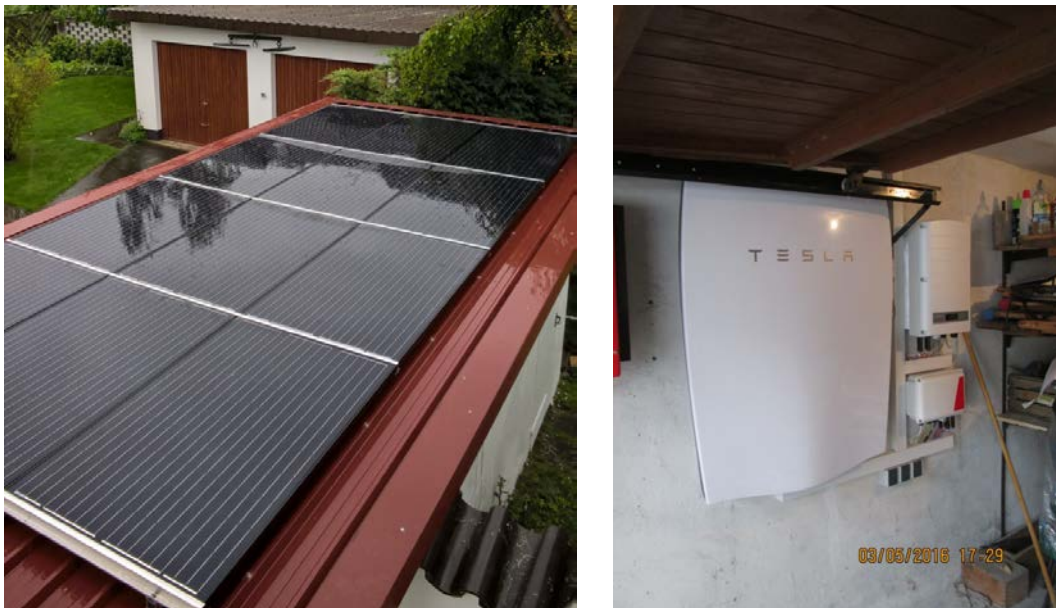
Figure 32: Right: The Tesla Power battery with integrated solaredge™ interface and inverter; left: The flat roof top mounted PV module as recently mounted in May 2016 during the trial period.
