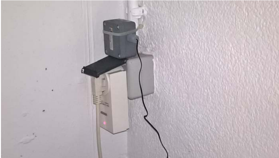
Figure 23: Smart plug as plugged into the socket to measure the consumption of the freezer and the radio transmitter of the T-sensor inside the freezer on top of the socket.
