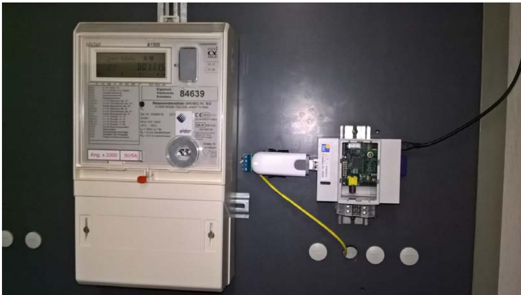
Figure 17: The picture of installation from the 17 th Oct. 2016, when the Raspberry PI-1 is again connected via S0-Interface with the A1500 Elster smart meter in the MV-LV distribution cabinet.
