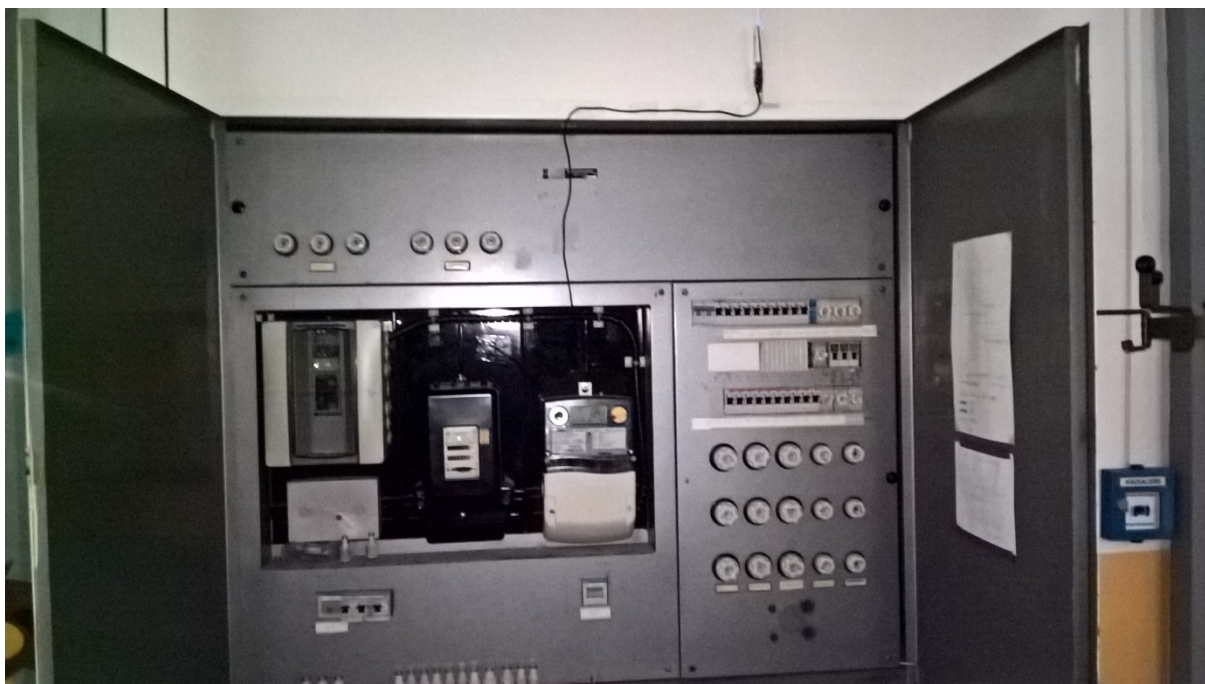
Figure 14: The opened electrical cabinet with the cable connection between the Raspberry PI, mounted in the left part of the picture and the UMTS data port which is mounted on top and outside the electrically shielded cabinet.
