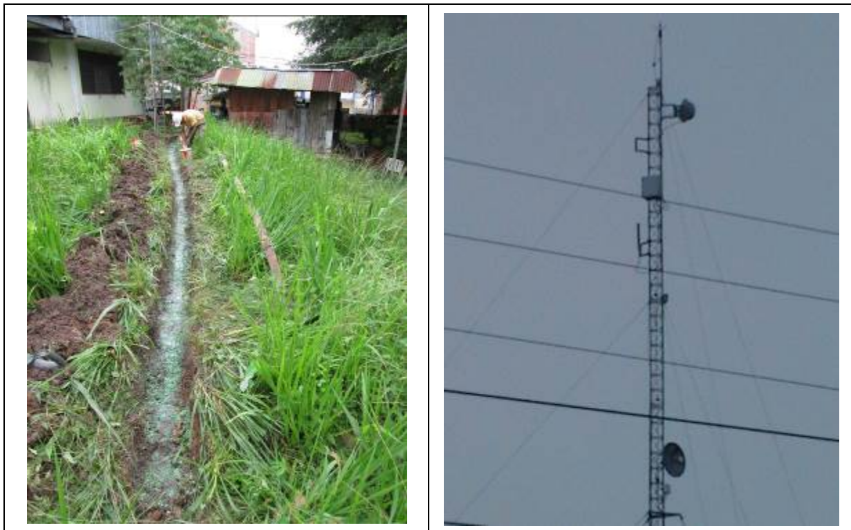
Figure 53: Upgrade of the grounding system and maintenance of the equipment used in the repeater located in Santa Gema Hospital
