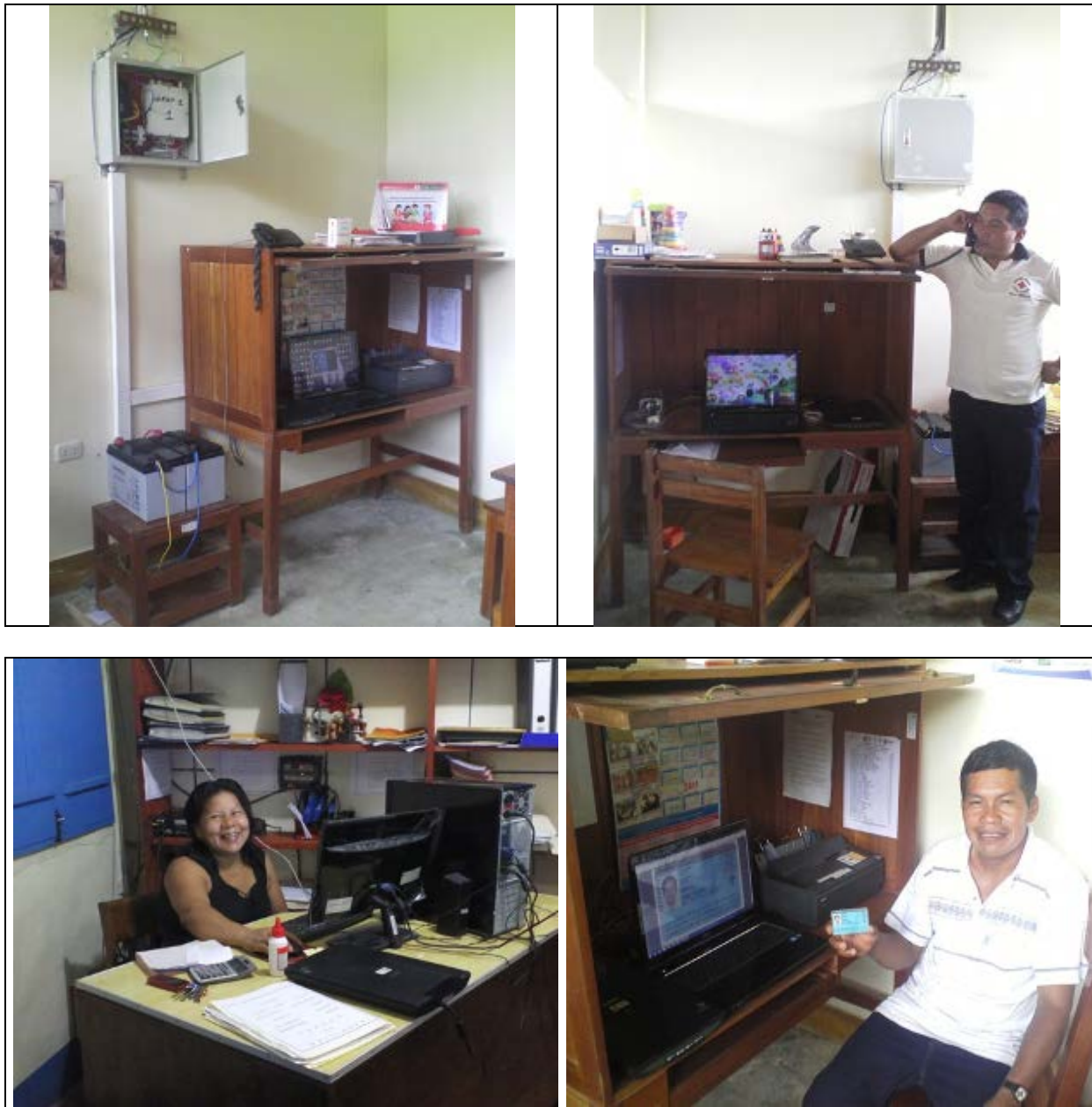
Figure 42: Torres Causana and Tempestad client stations (upper pictures); Napo Rural Telemedicine Network users (lower pictures)
