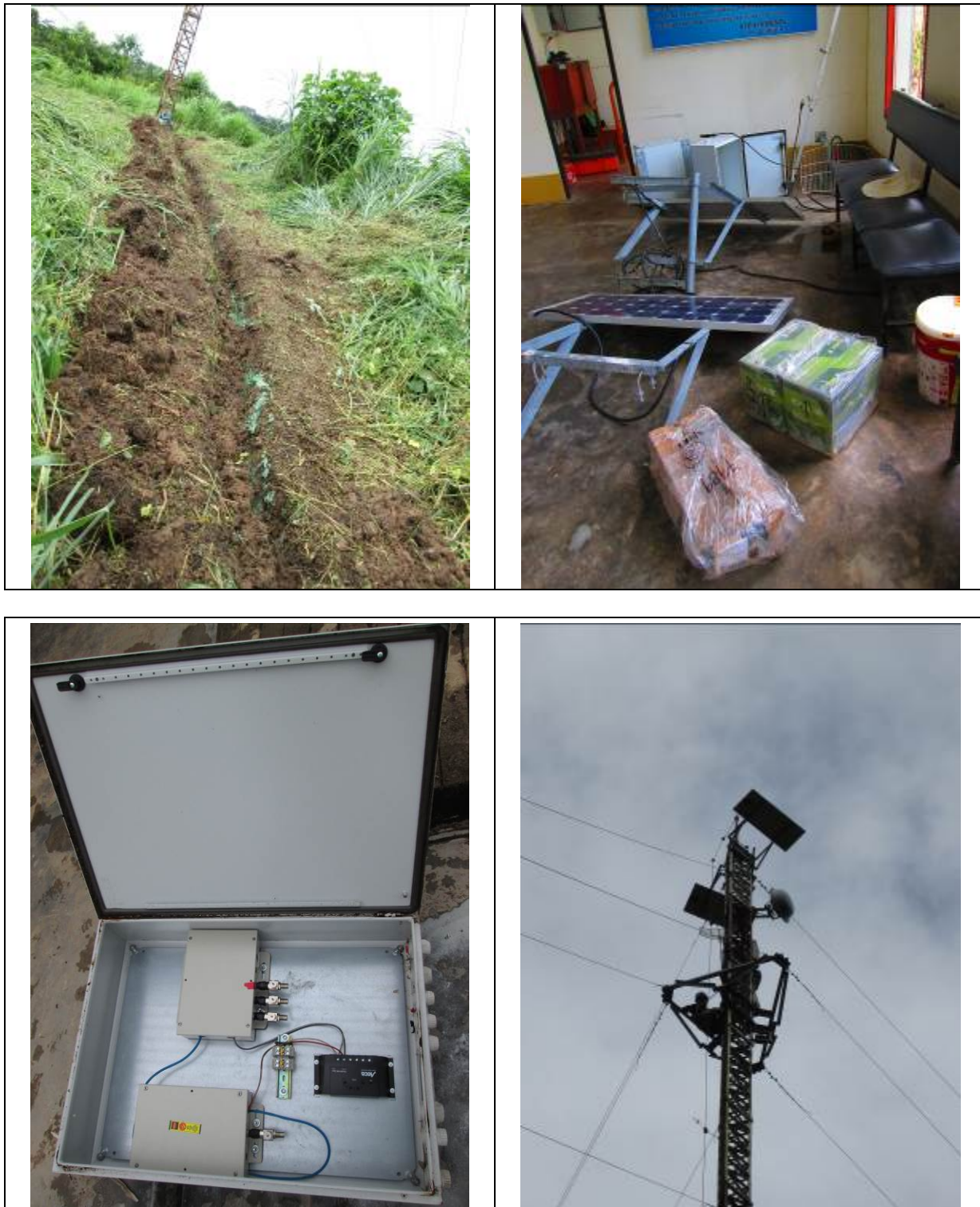
Figure 56: Upgrade of the grounding system and maintenance of the equipment used in the repeater located in San Gabriel de Varadero
