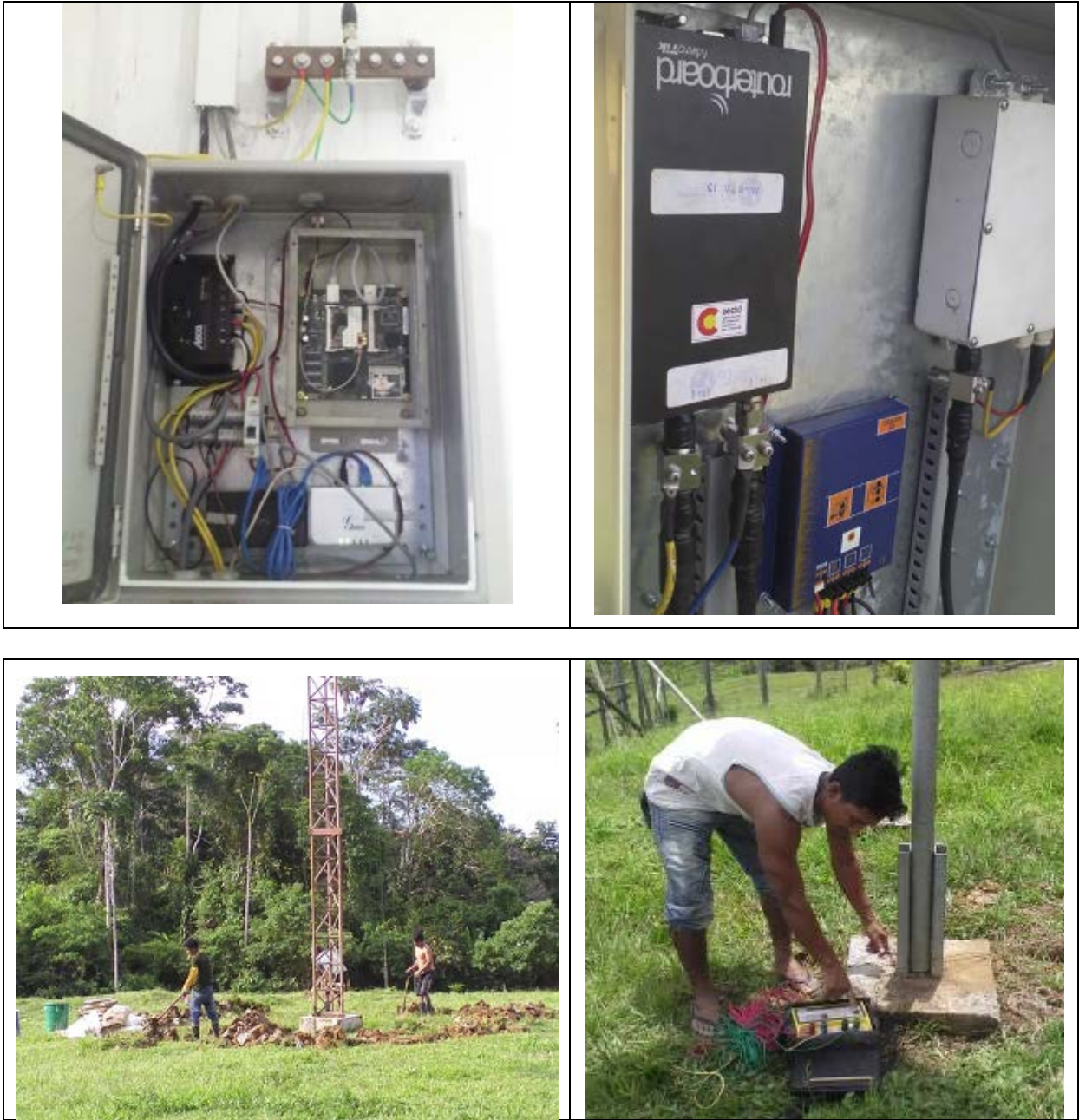
Figure 41: Client station (upper-left corner); repeater station (upper-right corner); Grounding system maintenance at the repeater station (lower-left corner); Grounding system maintenance at the client station (lower-right corner)
