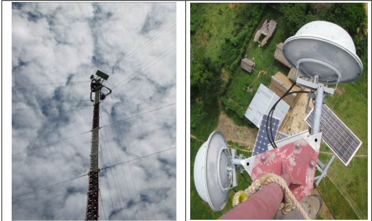
Figure 55: Maintenance of the equipment used in the repeater located in San Juan.
