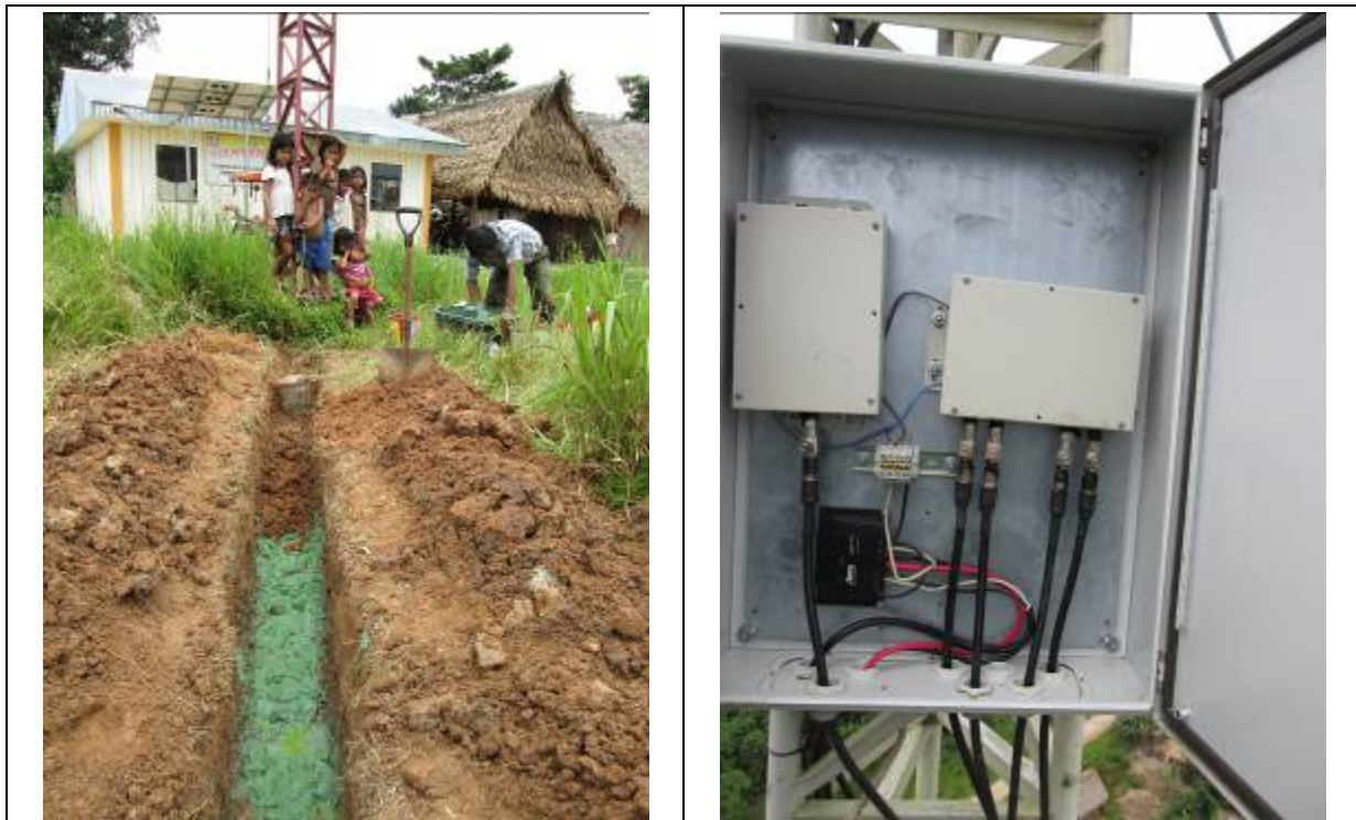
Figure 54: Upgrade of the grounding system and maintenance of the equipment used in the repeater located in Varadero
