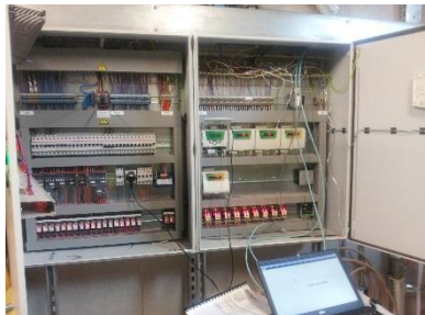
Figure 9-4 Control Panel CnaC
