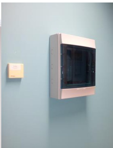
Figure 8-9: Installed Water Meter Enclosure at NUIG Office Area
