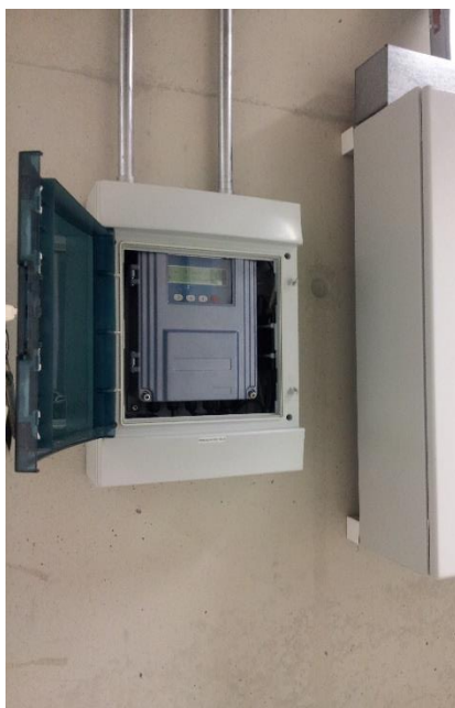
Figure 8-8: Installed Ultrasonic Water Meter at NUIG
